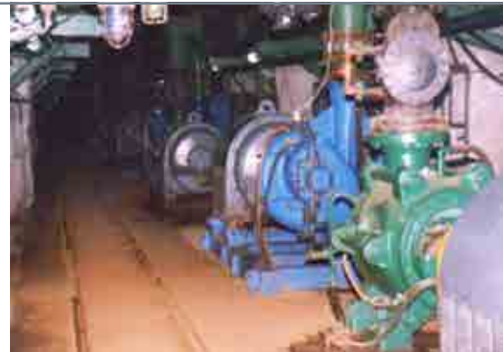
Bank of dewatering pumps.
