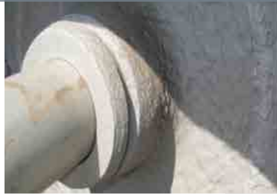
Condition of fan rotor after sandblasting.
