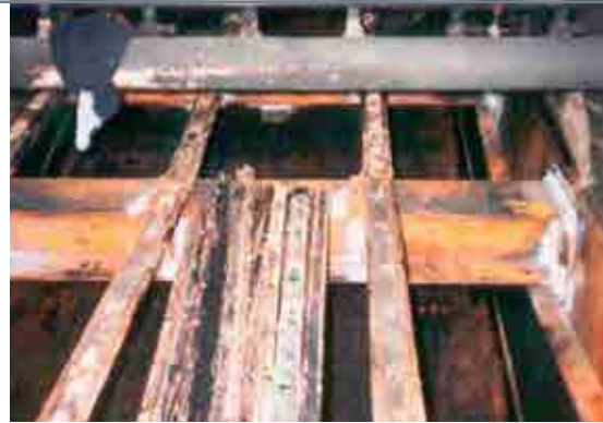
Damaged coal screen
