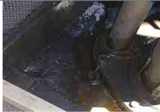
Pre-existing condition of concrete.
